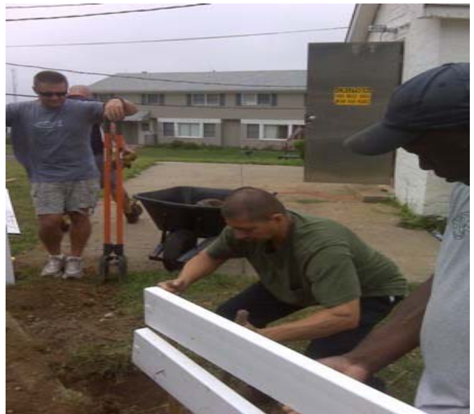
The crew working hard on the fence project at Sta Eaton’s Neck.
